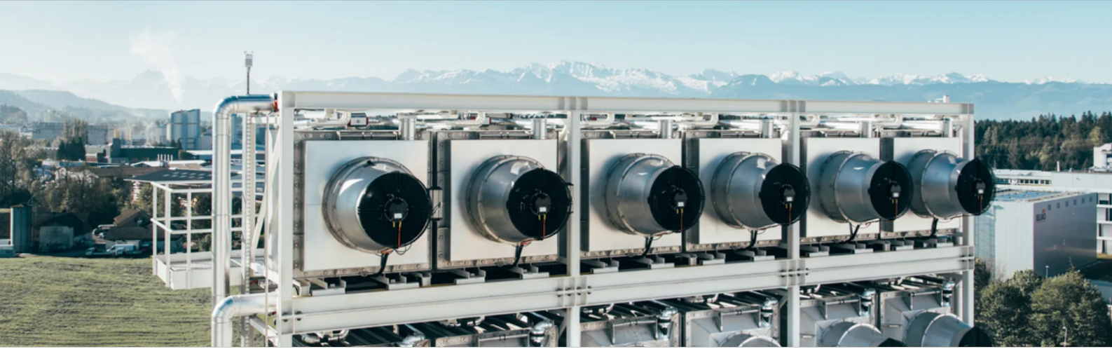
Climeworks DAC plant in Switzerland.
